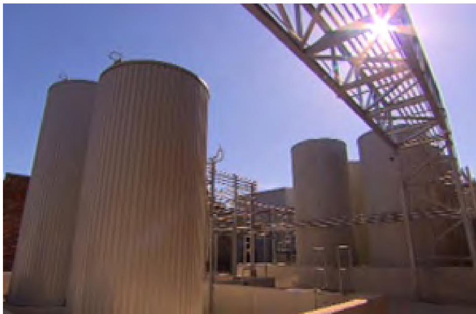
Plate 2.2. Agri Energy plant at Bootle, Merseyside for the recovery of useful products from used cooking oil.
