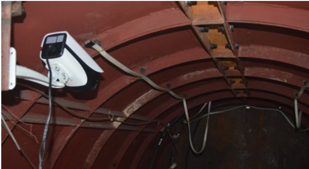
Photo 3 - Closed-circuit television (“CCTV”) system
