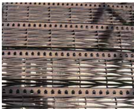
The existing catwalk stairs could be reused as a seating surface for benches.
