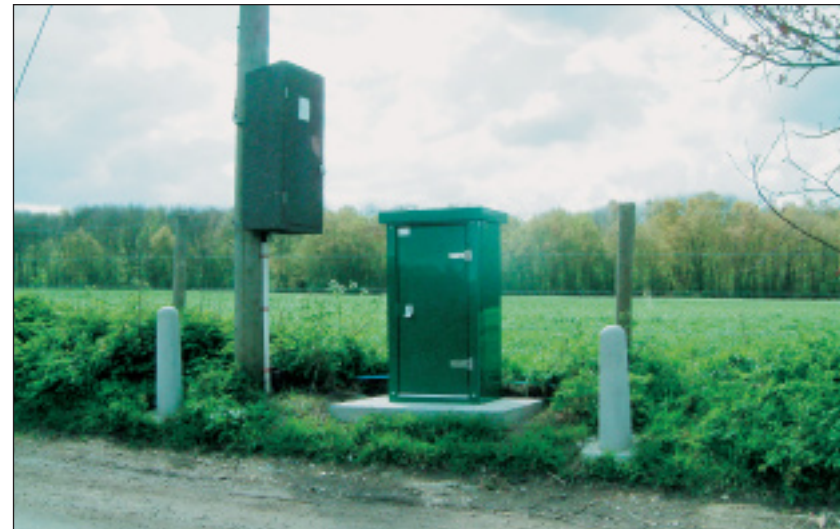
Far left: Poorly sited telecommunications mast
