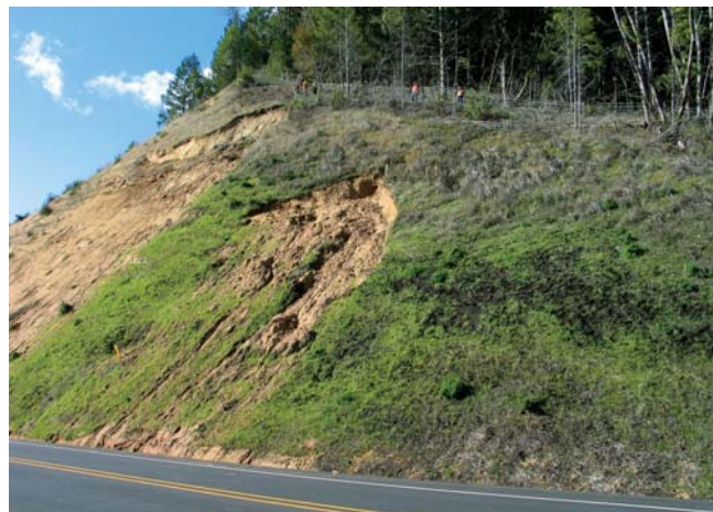
Figure 2 ~ This debris slide took place two years after construction, when grasses were fully established. To preclude these kinds of problems, revegetation should have the establishment of long-term plant communities, not just quick cover, as a goal.
