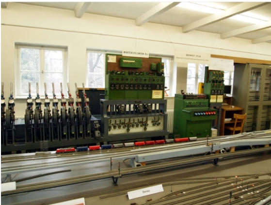
Old leverframe interlocking machines
