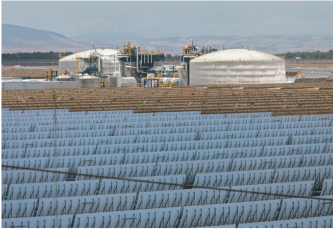
Figure 11.56 | Two-tank molten-salt indirect storage system at the 50 MW Andasol 1 parabolic trough plant in Spain. Source: Photo courtesy of Solar Millennium.
