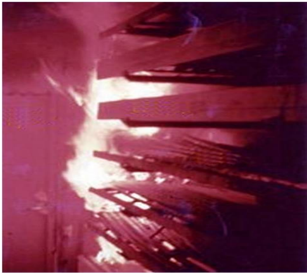
Burning insulation and sealant around electric cables at Browns Ferry in 1975. The fire started in a room located directly beneath the control rooms for the Unit 1 and 2 reactors. The cables connected controls and instruments in the control rooms with equipment throughout the plant.
