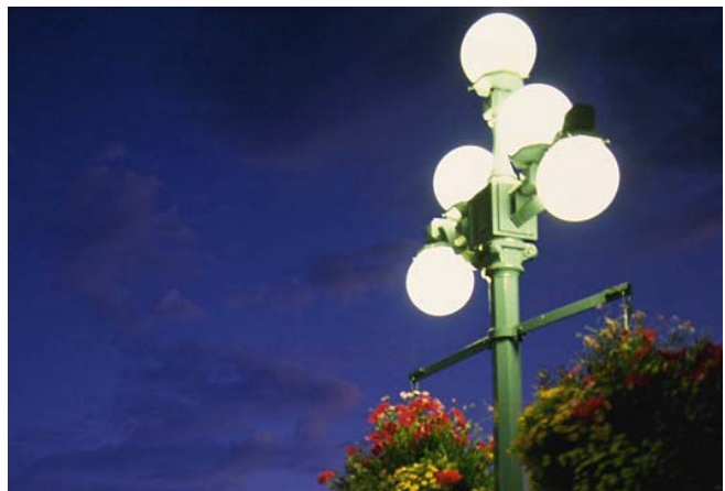
Streetlights with five fixture heads per pole
