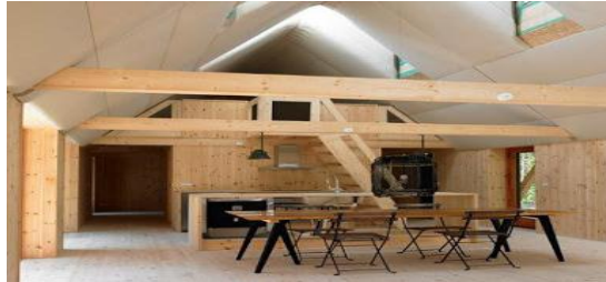
Fig.1.1 Insulation of seaweed fibres between the rafters of pitched roofs
