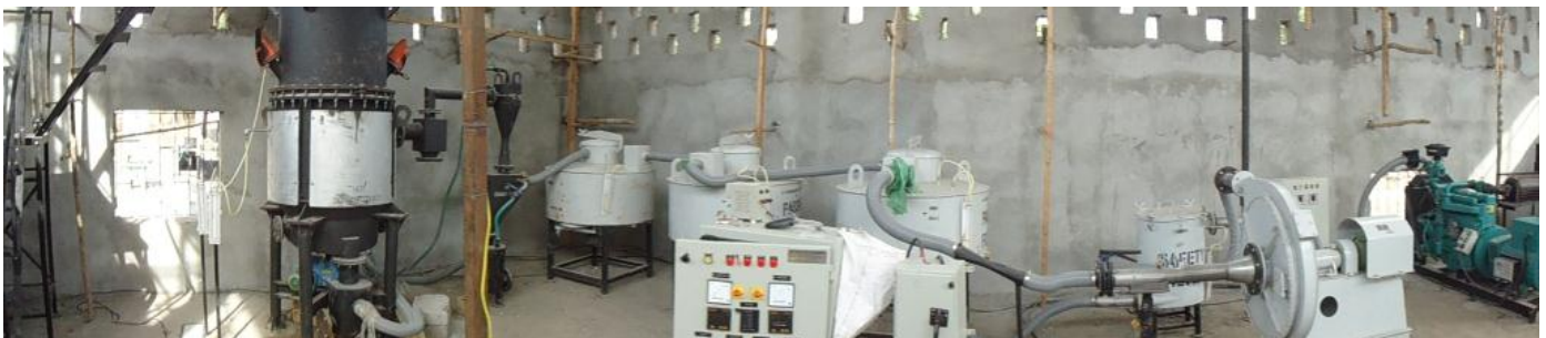
Figure 2. Photograph of the Kychom gasifier assembly.
