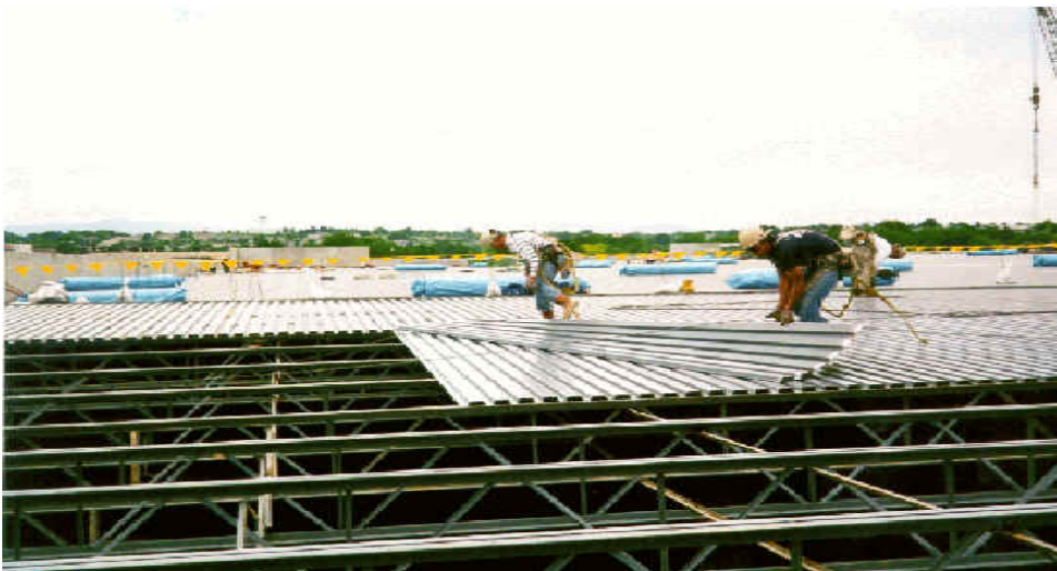
Figure 4-18. Leading edge work. (Source: OSHA fall protection guidelines).
